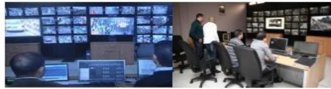
Fig 1: Base of command supervision
